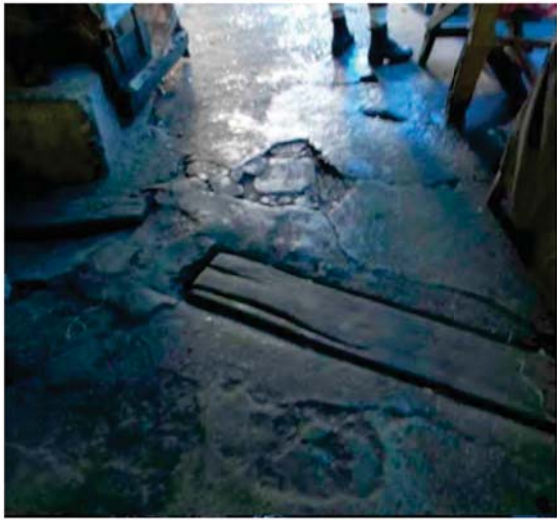
Image 12 Poor surface and makeshift drain covers
